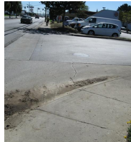
Figure 3: No detectable warnings at bottom of curb
