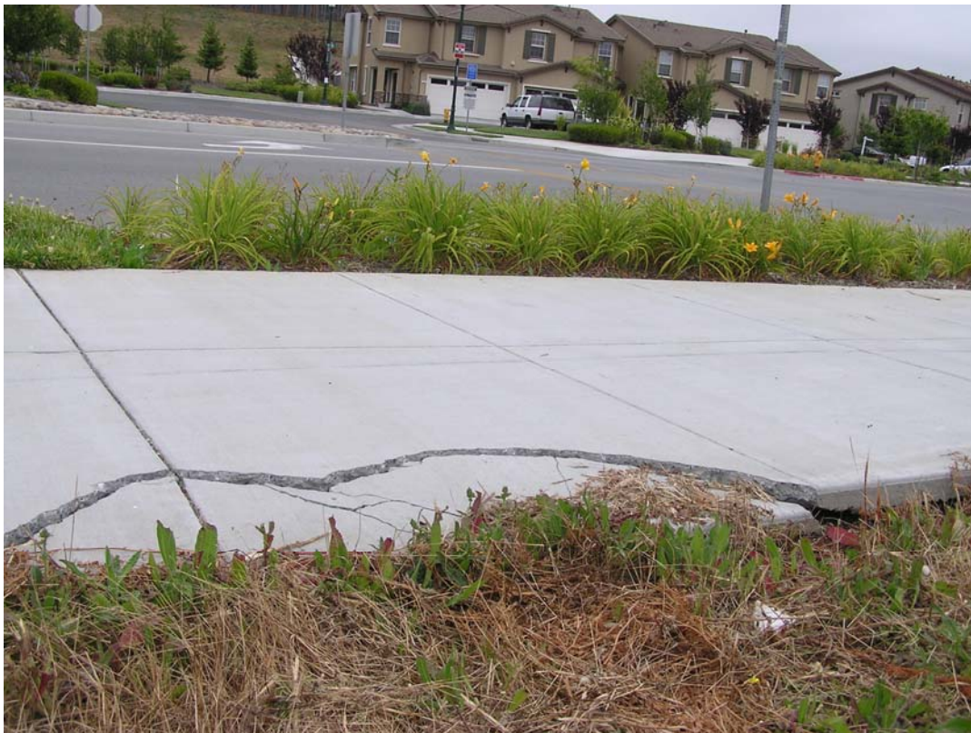
Figure 6. Crack in new sidewalk.
