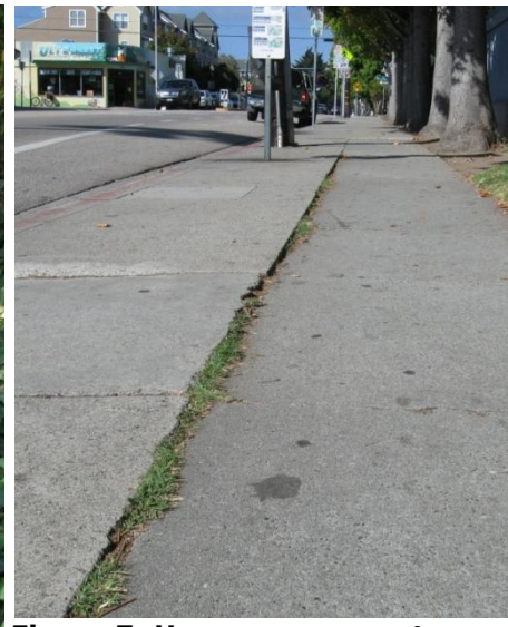
Figure 7: Uneven pavement, difficult for vision and mobility impaired pedestrians
