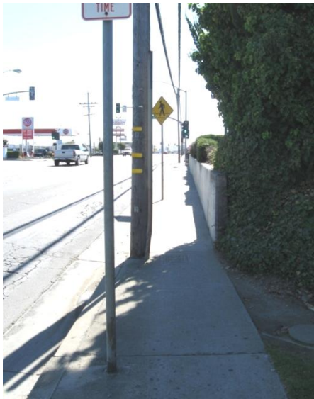
Figure 5: Fixtures in sidewalk encroach in travel path
