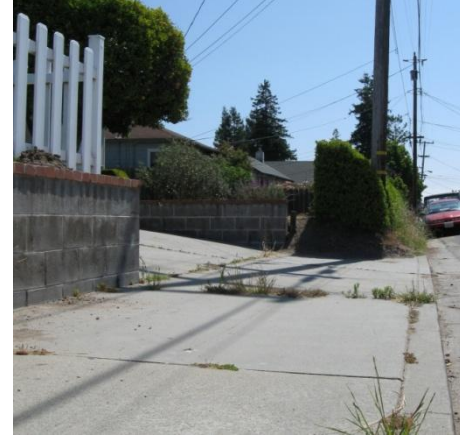
Figure 11: Driveway slope not even with sidewalk
