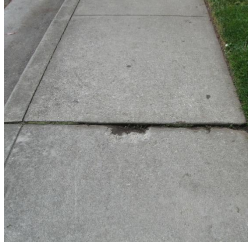
Figure 10: Rough and uneven sidewalk surface is tripping hazard
