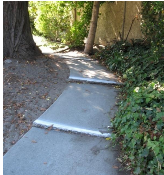
Figure 6: Sidewalk uplift due to tree roots
