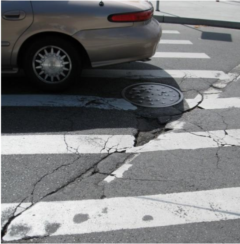
Figure 9: Rough and uneven pavement in crosswalk
