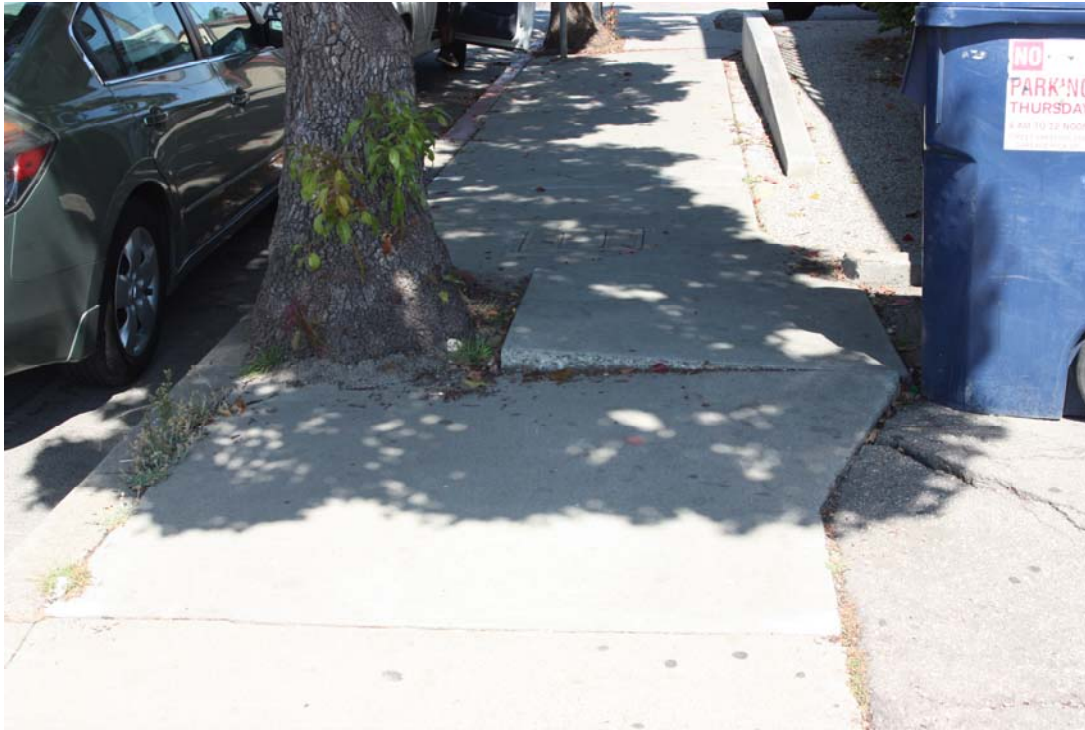
Figure 1. Sidewalk uplift due to tree roots.
