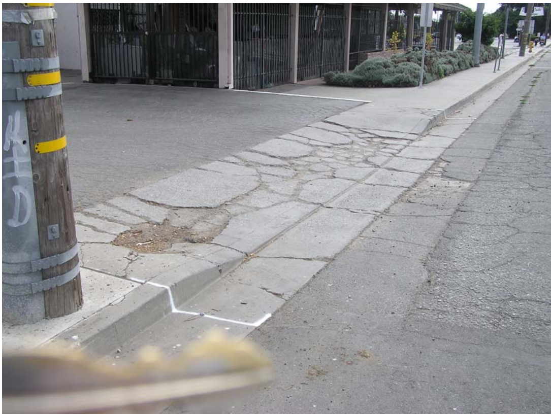
Figure 2. Large cracks in driveway.
